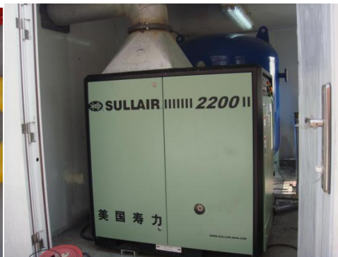
air compressor and air tank
