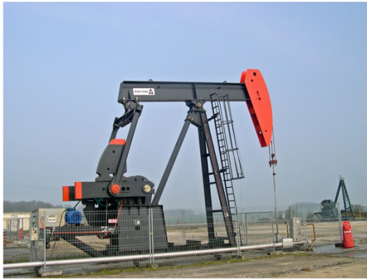
Beam pumping unit
